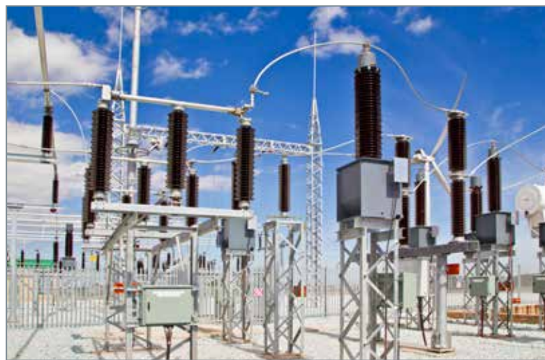
The company has completed six separate grid connection projects totalling 127 MW.
